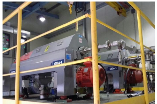
Power Plant water application
