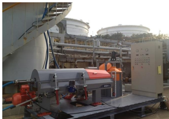
Chemical waste water application
