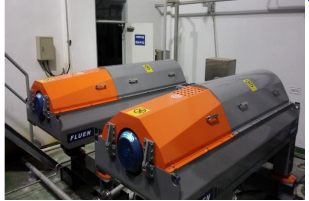
Sewage water application
